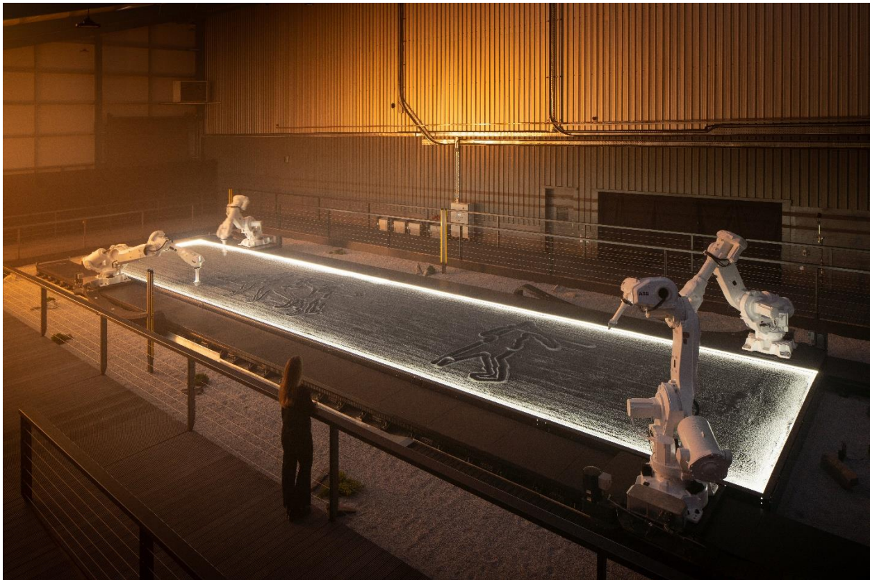
Test build of The Constant Gardeners , 2021, photo by James Medcraft, courtesy of Jason Bruges Studio
